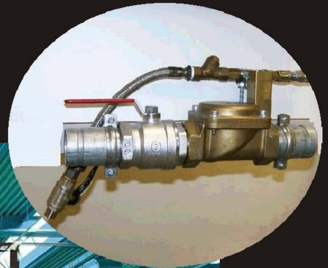
Control Valve Unit
